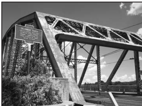
DECK STUDY: A $30,000 analysis to potentially replace the open metal grid deck system of the 1939 Port Jervis, NY-Matamoras PA Bridge will be funded this fiscal year ending March 31, 2021. (UDC Photo by Laurie Ramie)
