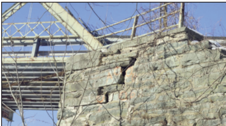
MOVING MASONRY: Engineers cite cracks in the New York abutment of the Skinners Falls-Milanville Bridge as problematic. (UDC Photo by Kerry Engelhardt)
