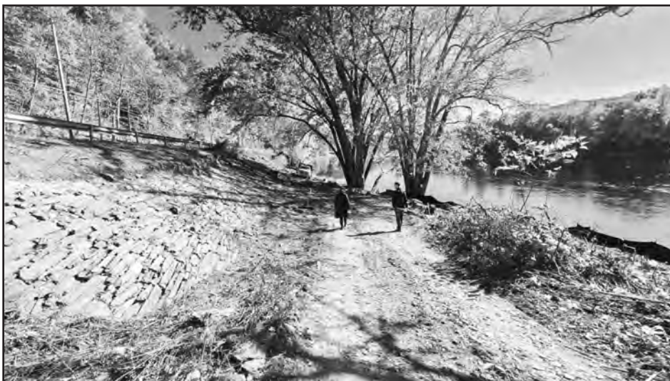
NYS ACCESS CLOSED: The Highland River Access located along NYS Route 97 between Barryville and the Roebling Bridge closed to public use October 3 until Spring for construction work by Wheat and Sons, a contractor hired by Sullivan County to replace the existing gravel parking with pervious pavement, install bioswales, restore native plants, regrade the access with a more gently sloping and stabilized path down to the boat ramp, and install signage. Sullivan County received a $250,000 grant from the Delaware Watershed Conservation Fund, $100,000 from the State of New York, and pledges for $305,345 worth of in-kind services by the Town of Highland, NYS Department of Transportation, Department of Environmental Conservation, and National Park Service. Above, Sullivan County Senior Planner Heather Jacksy and Barryville activist John Pizzolato walk by a D&H Canal era stone wall that was exposed during the site work and will be left intact. (UDC Photo by Kerry Engelhardt)
