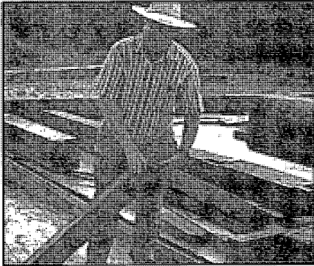
The Cochecton Railroad Station is on the move as Woody Schlagel, President of the Cochecton Preservation Society, and a host of volunteers begin reconstructing the historic building on its new foundation and new location just off NYS Route 97. In 1993, the UDC provided the original seed money to get this project started in the form of a Technical Assistance Grant. Photo: The River Reporter
