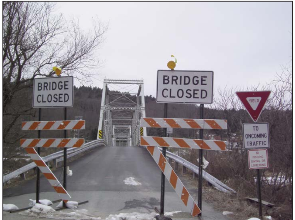
SIX-MONTH DETOUR: The Pennsylvania Department of Transportation closed the Skinners Falls, NY-Milanville, PA Bridge on Dec. 15, 2012 after an inspection revealed safety concerns with support beams. It is due to reopen by May 3 following repairs. (UDC Photo by Laurie Ramie)
