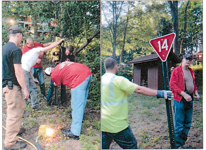
At left, volunteers drive in support posts for the numbered signs, shown at right, installed along the bank of the Lackawaxen River.
